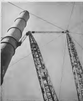
STACK, derrick and cables form symbol of job against the sky. STACA, grua y cableana ta forma simbolo di un trabao contra halturna.
